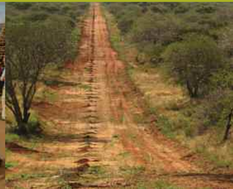
Fence post holes dug by hand for the Mkomazi Rhino Sanctuary Extension
